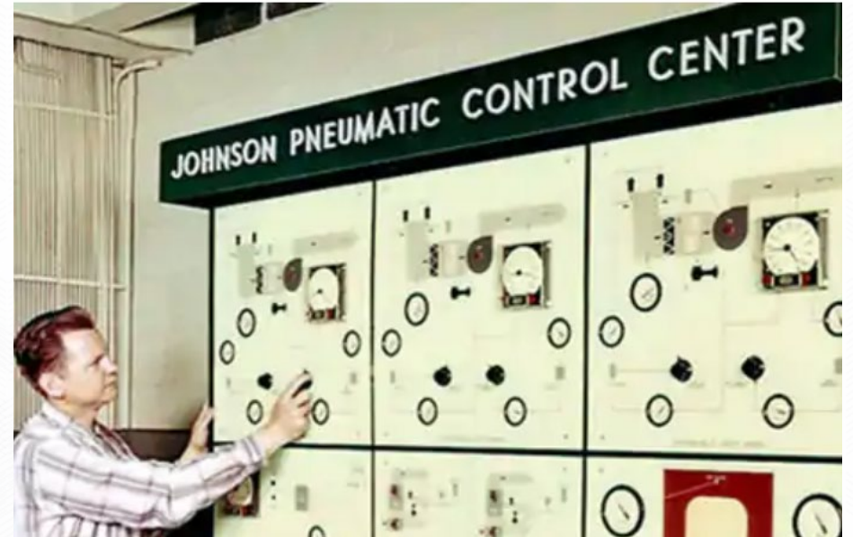
Source: Johnson Controls Inc.
