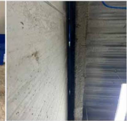
Leakage at temporary seal of exterior gym wall
