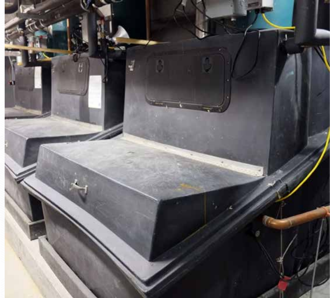
Composting Toilets @ Brock Environmental Center
