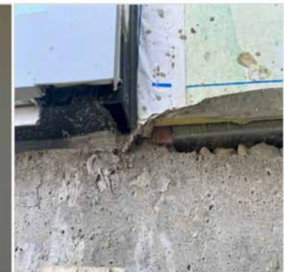
Leakage at bottom corners of storefront windows
