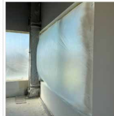
Corner windows missing gaskets causing leakage
