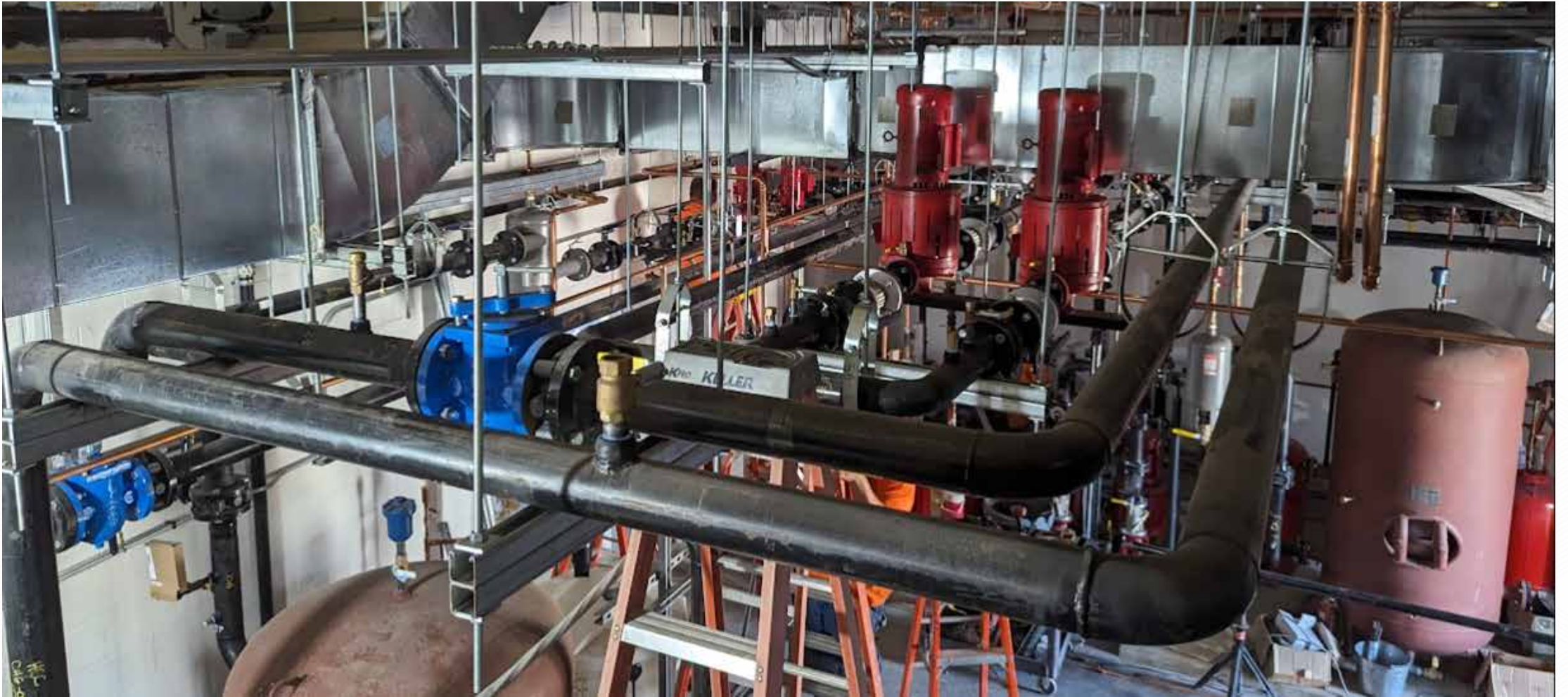
Mechanical Room @ HCC Agricultural Complex
