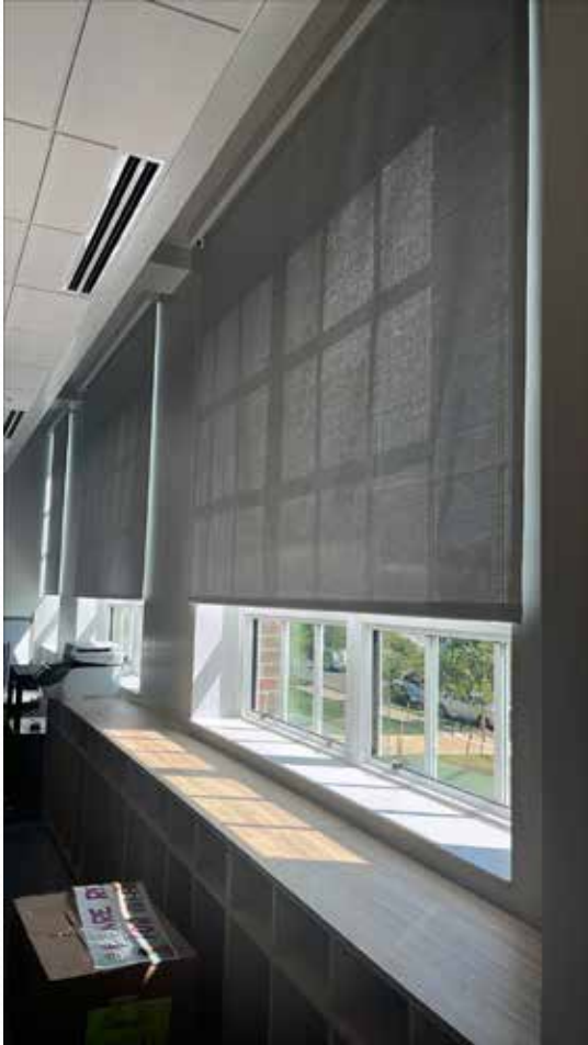
Daylight-controlled blinds stuck halfway, unresponsive to flashlight
