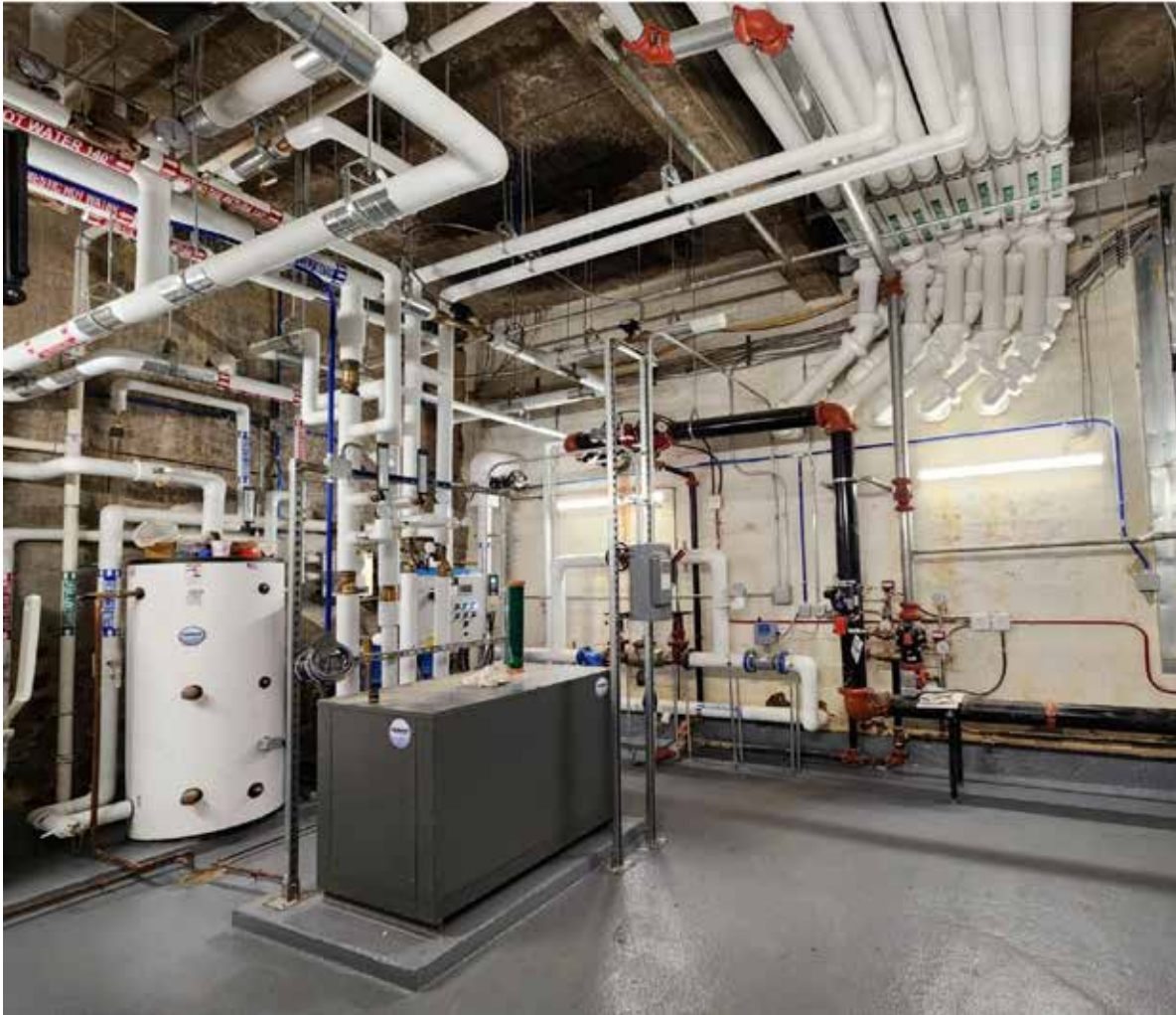
ASHP DHW @ Raymond Elementary
