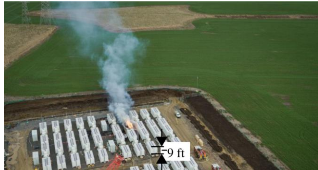
Victoria Big Battery (2021) Image courtesy of Fire Rescue Victoria [4]
