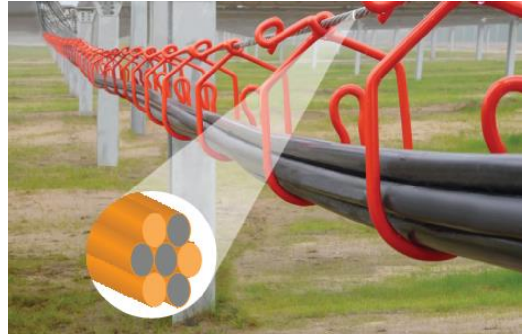
Example messenger wire system (courtesy of CAB Products).
