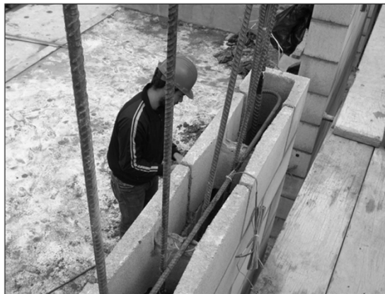
Shear reinforcement in special walls must be anchored around end vertical bars with a hook TMS 402 §7.3.2.6(f)
