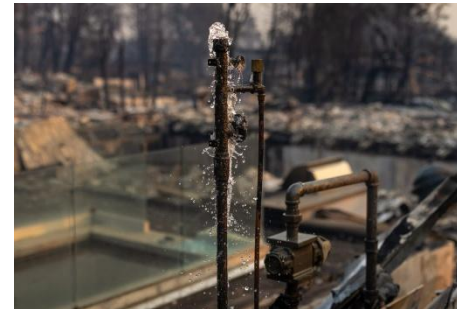
Leaks at Destroyed Structures
