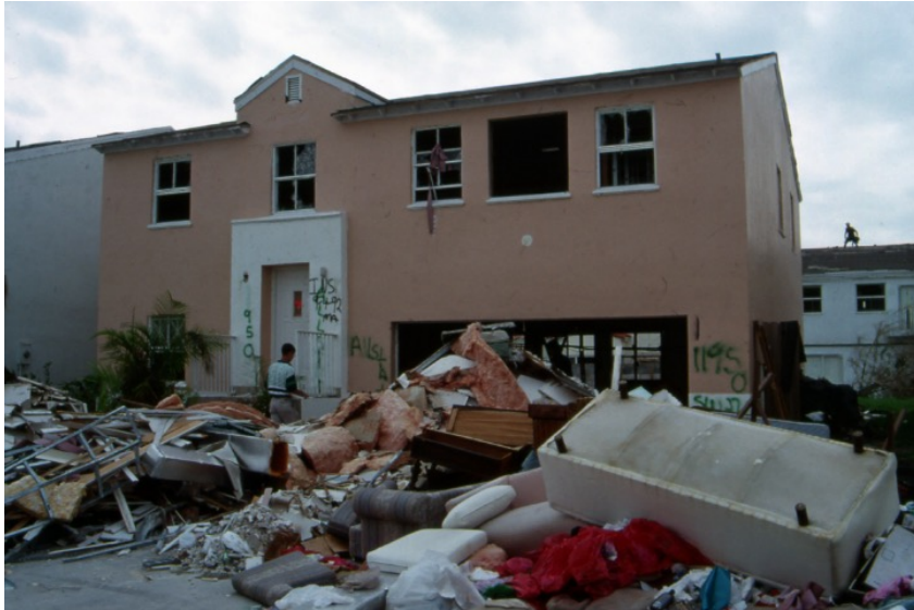
Extreme Wind-Driven Rain Hazard (Tropical) – Hurricane Andrew, 1992 (~600 yr MRI wind event); Contents water damage in South Florida due to breach of building envelope
