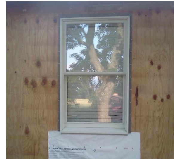
Typical Wind-Driven Rain Hazard Exposure (non-tropical, t-storms, etc.); 35-year old one-story building; only minor water staining below window with no WRB, flashing, or bedding sealant
