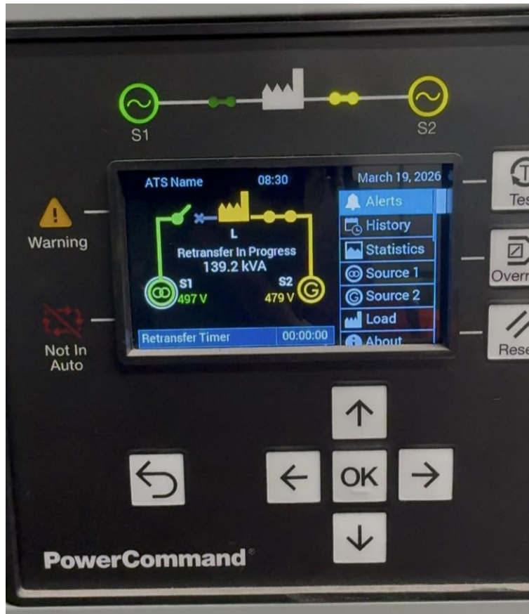
Transfer from (Utility Power) to Source 2 (Generator) happened in under 8 seconds.
